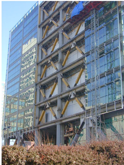
Fig. 7. Photos of: (a) Wallace F. Bennett Federal Building; (b) view of building without cladding showing installed buckling-restrained braces (Photos courtesy of SIE Corp.)
