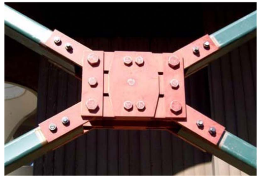
Fig. 10. Photos of (a) patient tower; (b) closeup view of installed cross-brace friction dampers [Reprinted from Shao et al. (2006), with permission from the Earthquake Engineering Research Institute]
