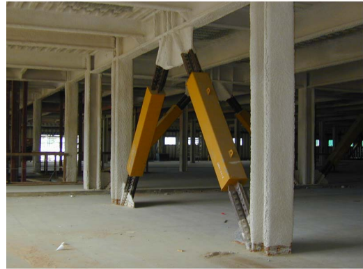
Fig. 8. Photos of: (a) Santa Clara Medical Center Hospital under construction; (b) closeup view of installed buckling-restrained braces (Photos courtesy of SIE Corp.)
