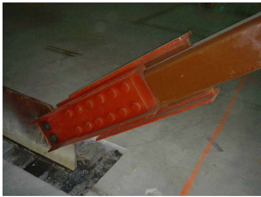
Fig. 9. Photos of (a) Monterey County Government Center showing precast concrete panel cladding; (b) closeup view of installed friction damper [Reprinted from Chang et al. (2006), with permission from Earthquake Engineering Research Institute]
