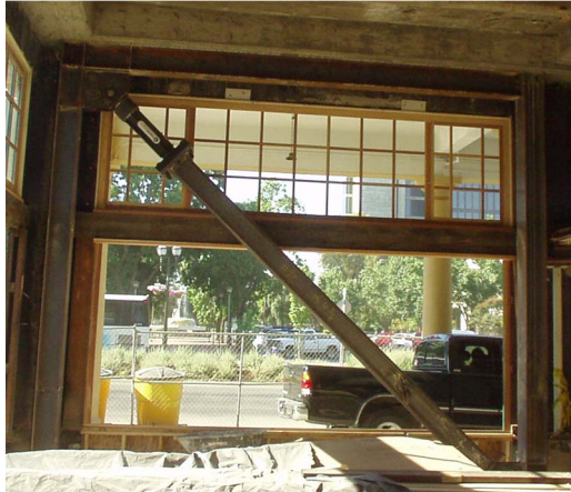
Fig. 5. Photos of: (a) renovated Hotel Stockton; (b) view of installed fluid viscoelastic damper (Photos courtesy of Miyamoto International, Inc.)
