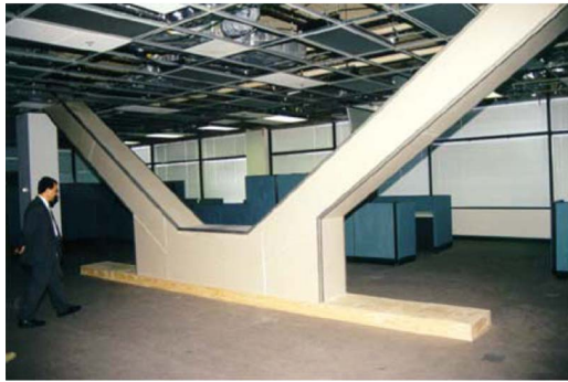
Fig. 11. Photos of: (a) LAPD Recruit Training Center; (b) view of chevron brace assembly containing viscoelastic damper at floor level (Photos courtesy of The Crosby Group and SIE Corp., respectively)
